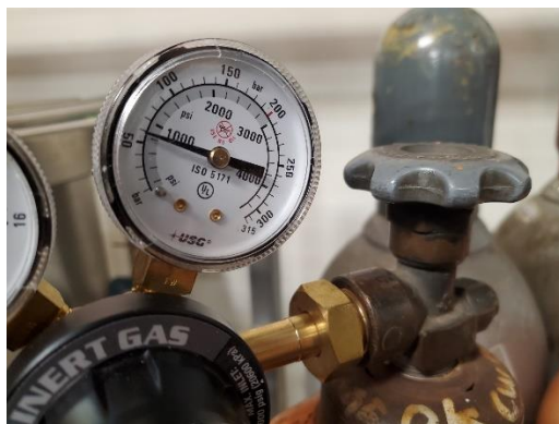
Figure 7-9: Main Valve Tank Pressure
