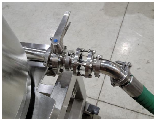
Figure 7-12: System Outlet Valve in Closed Position
