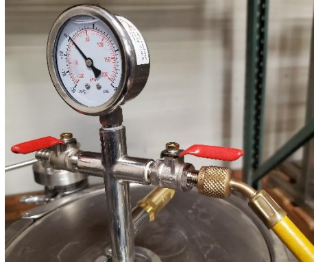
Figure 7-13: Dip Tube Manifold Ball Valve in Open Position
