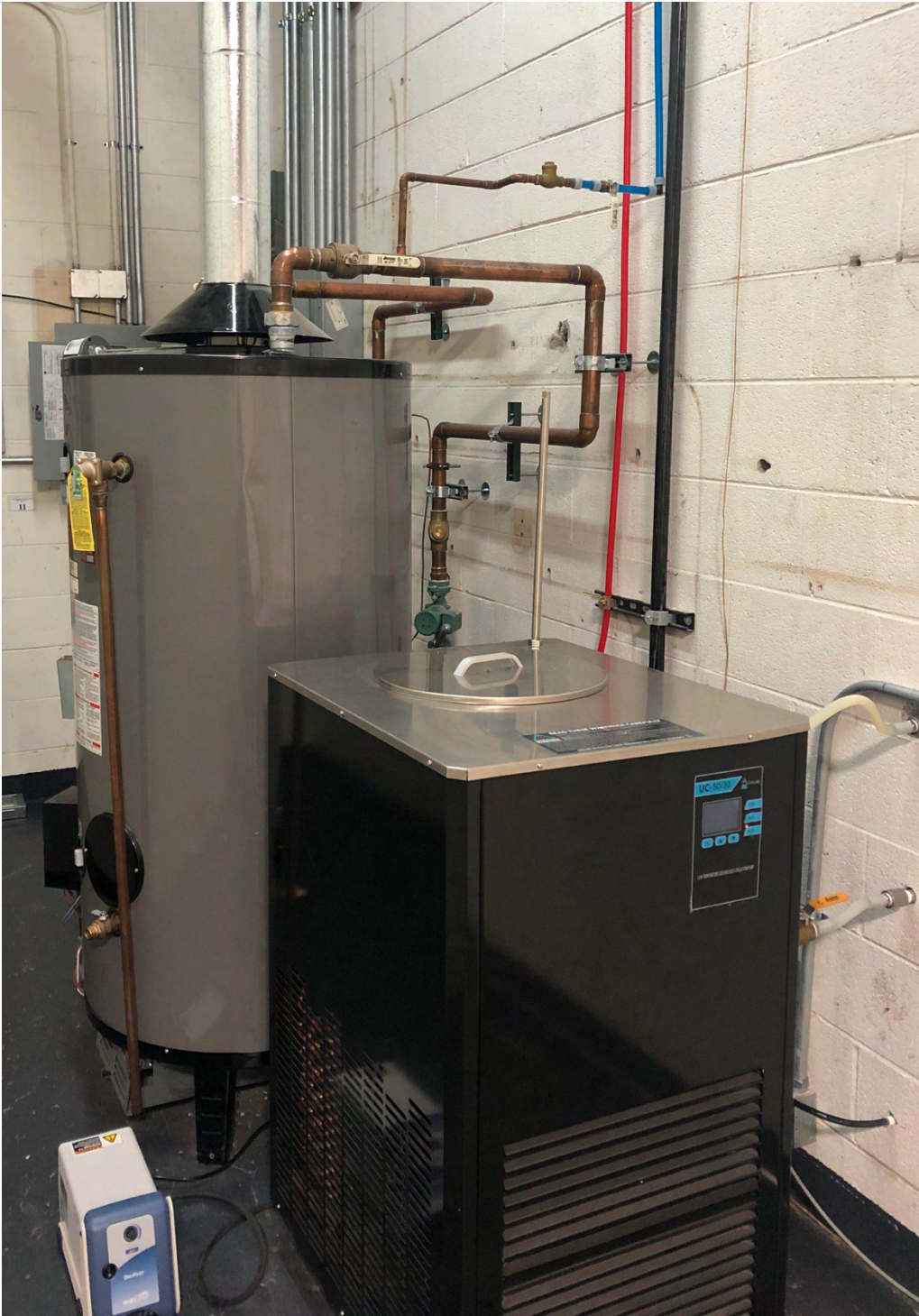
Boiler/Water Heater 100 Gallon
