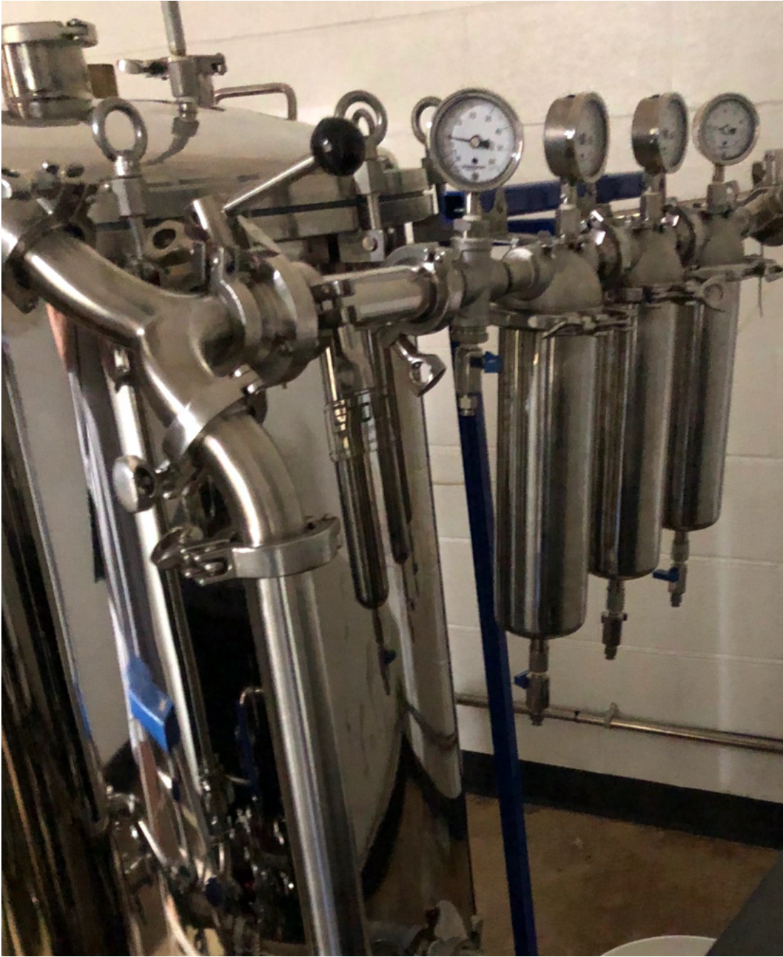
3 Stage Filter Skid with pressure valves
