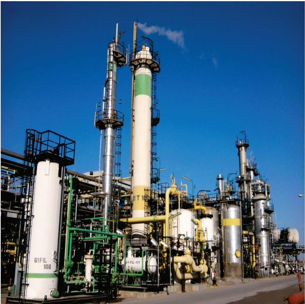
Figure 01: 6P LNG unit with the new modifications
