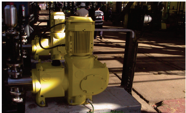
Figure 12: new washing pumps 61 P101A/B
