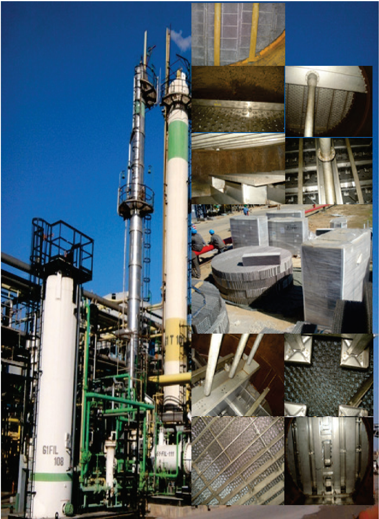
Figure 10: Substitution of the acid gas removal column 61T101 internals by structured package
