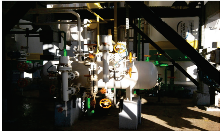
Figure 13: new drain collector drum 61D106
