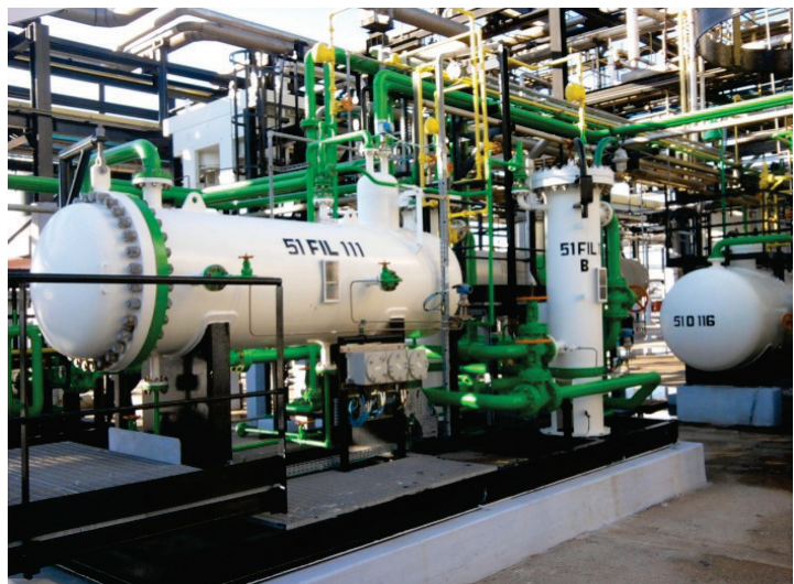
Figure 14: new filters 61FIL111 and 61FIL110 A/B
