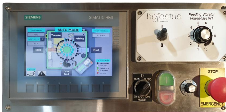
Emergency stop PB on control panel
